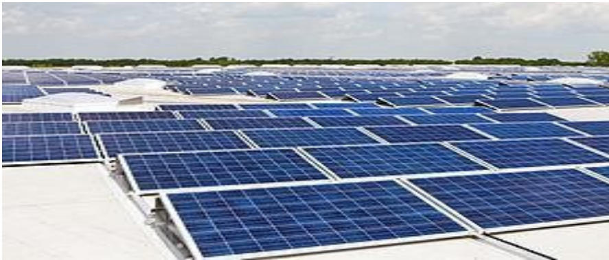
Fig. 1. Solar modules arrangement
